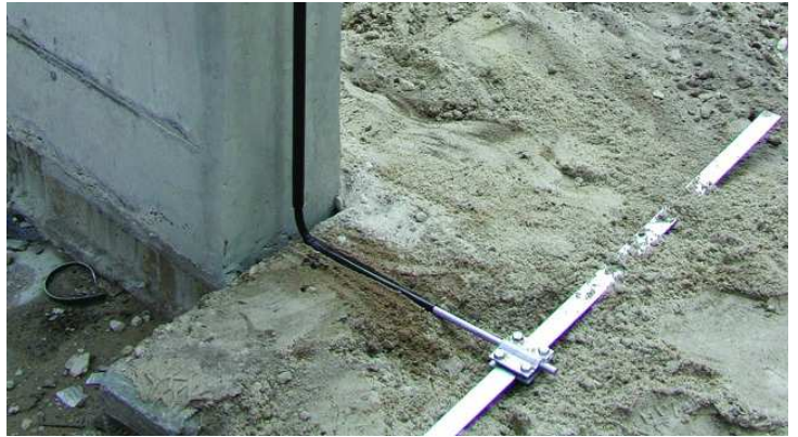
Connection between down conductor and earthing system
