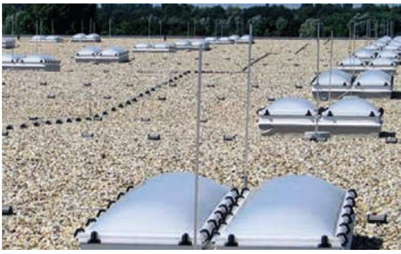
Lightning protection on flat roof
