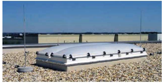
Small air-termination rods on flat roof
