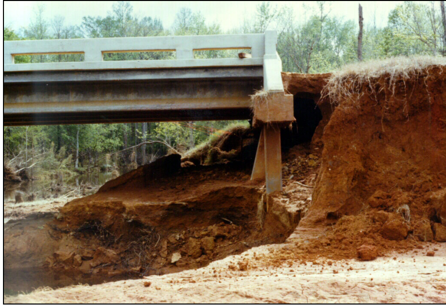
Figure 2.11.0.1 Example of damaged support abutment due to scour at the bridge opening (courtesy of USGS)
